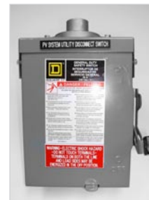
AC Disconnect Switch
